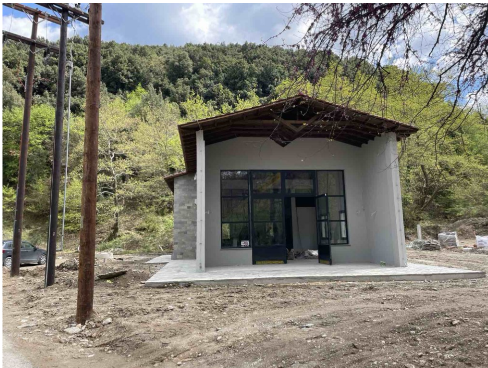
Figure 2.50 Photo of Hydropower station.
