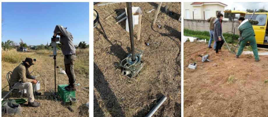
Figure 5.11 Drilling in the vadose zone for the establishment of the ceramic cups.
